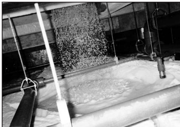
The ice slurry exiting a generator drops directly into the storage tank. If required, the ice slurry can be pumped to one or more tanks located remotely from the ice generator.
