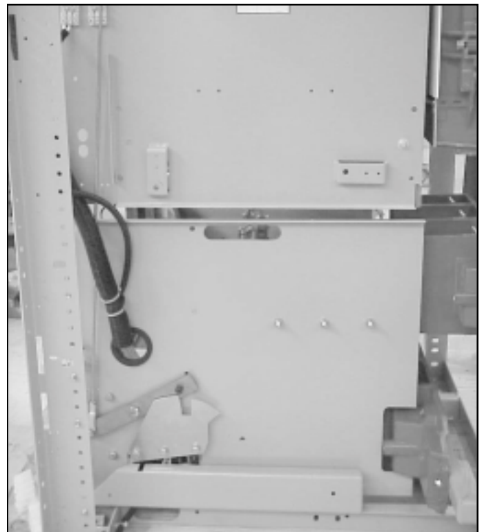
Fig. 8 Contactor Open, Interlock Neutral
