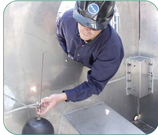
The water level control is easily reached from the access door
