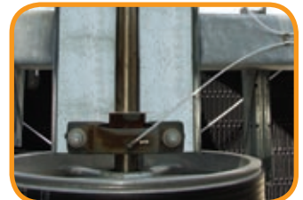
Grease fittings at the bearings
