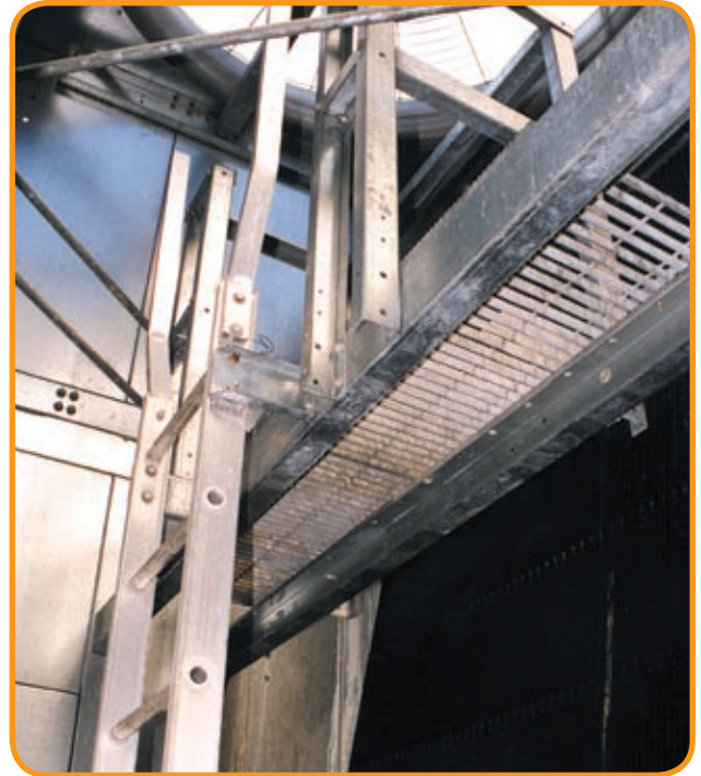
Internal ladder and service platform
