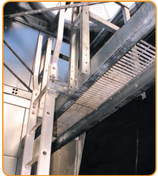
Internal ladder and service platform
