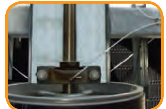
Grease fittings at the bearings
